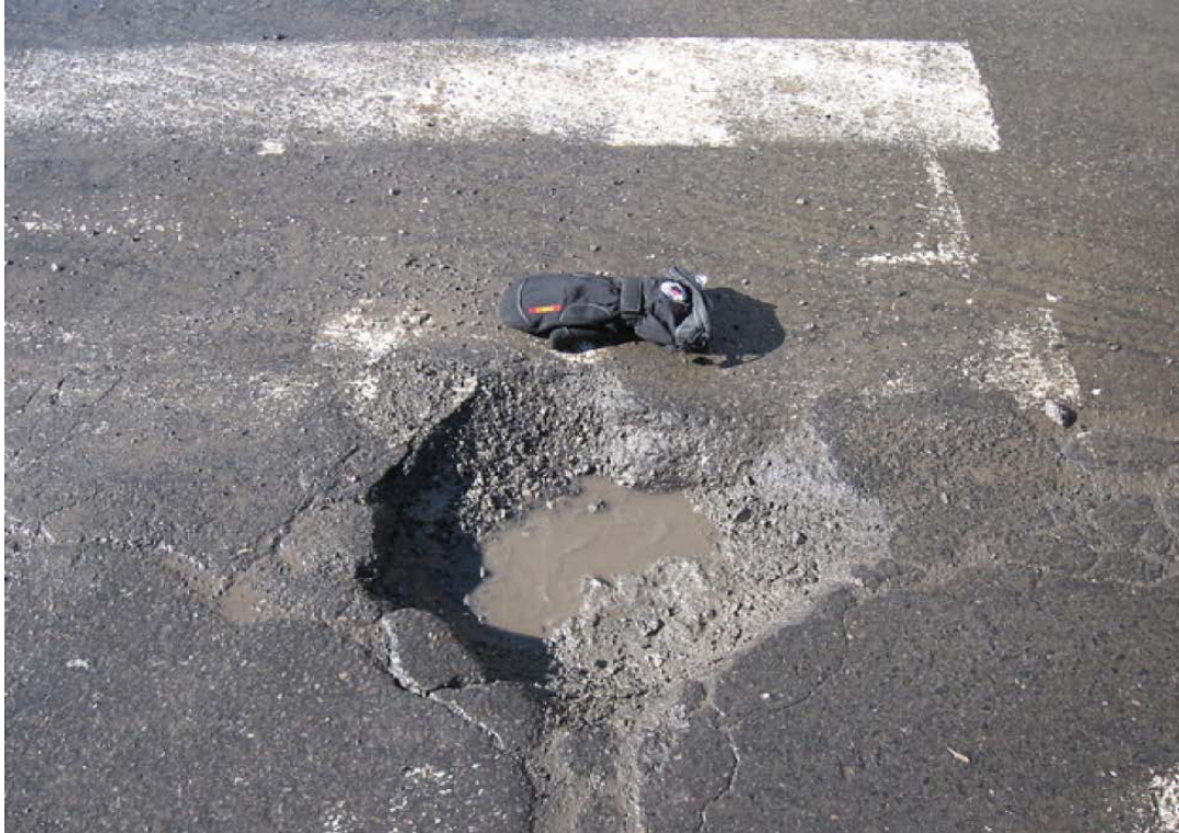
File: Pothole.jpg. (n.d.). [Digital image]. Retrieved from https://commons.wikimedia.org/wiki/File:Pothole.jpg
