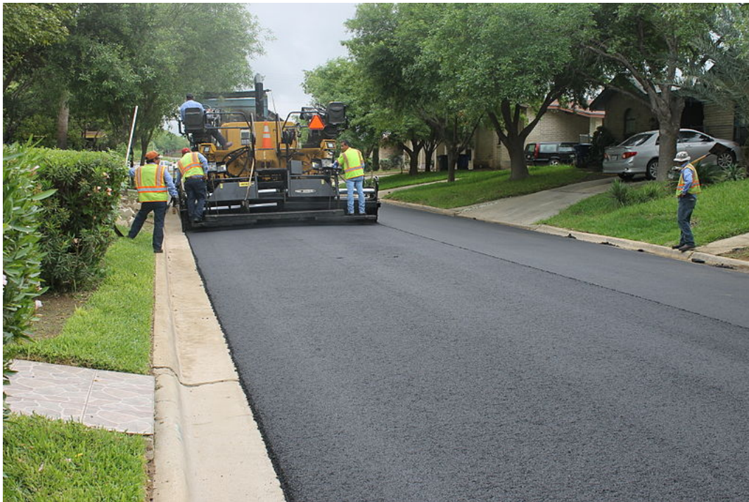
File:Street paving in Laredo, TX, 2015 IMG 5515.JPG. (n.d.). [Digital image]. Retrieved from https://commons.wikimedia.org/wiki/File:Street_paving_in_Laredo,_TX,_2015_IMG_5515.JPG
