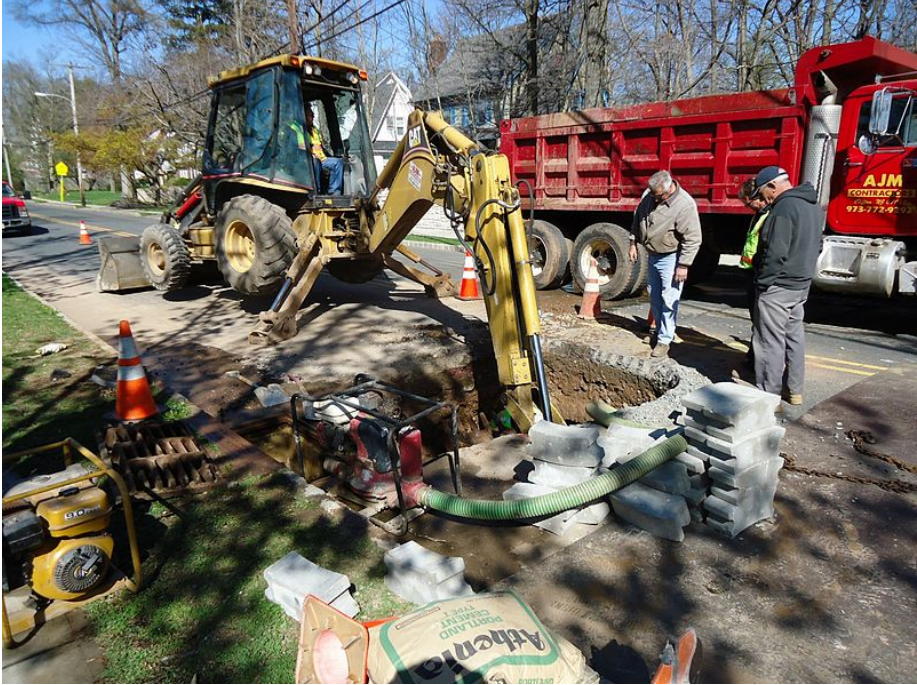
File: Road repair digging beneath street.jpg. (n.d.). [Digital image]. Retrieved from https://commons.wikimedia.org/wiki/File:Road_repair_digging_beneath_street.jpg
